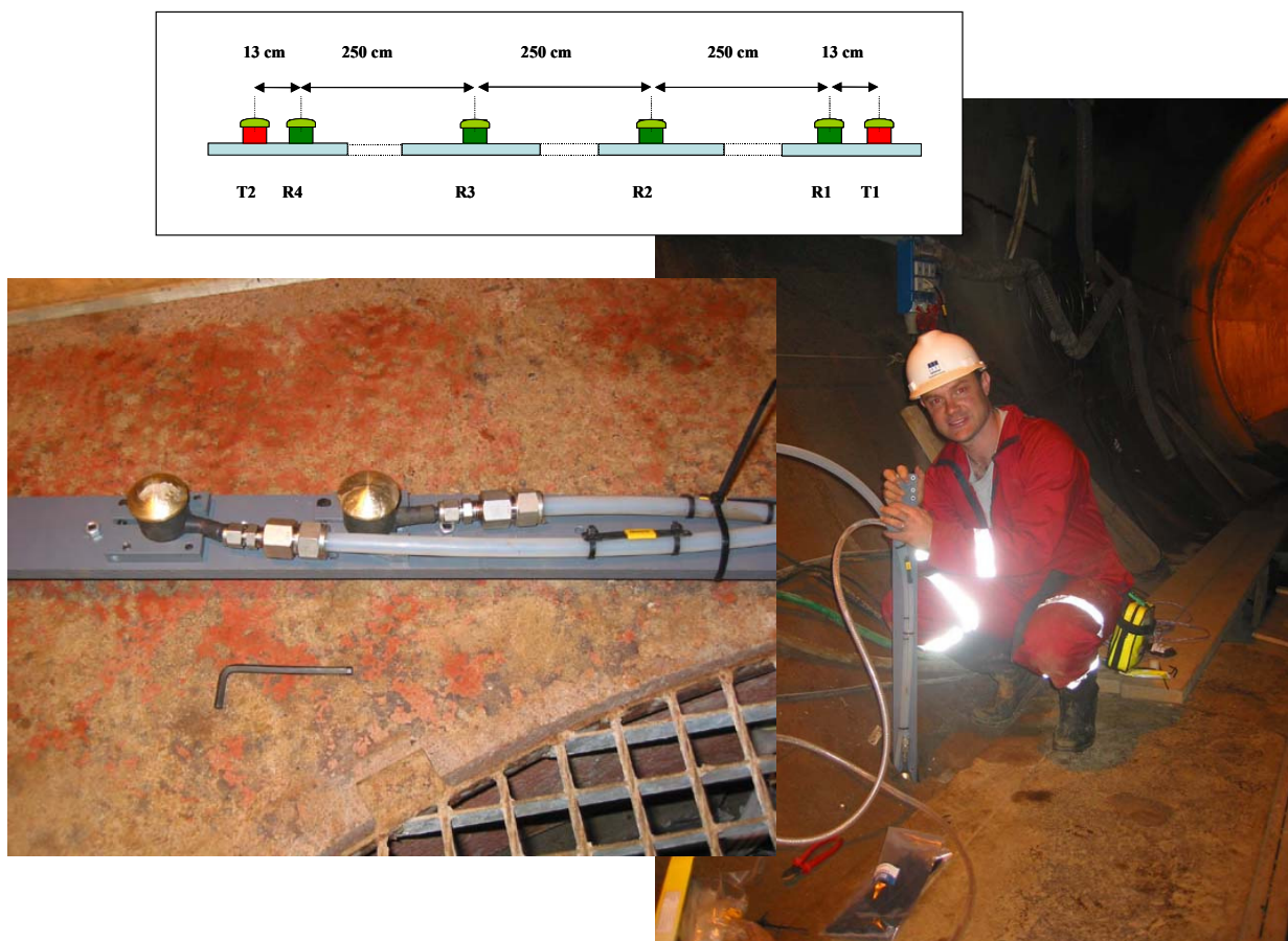
Figure 4-13: Top: Schematic diagram of the locations of all transducers on a single frame. Left: Photo of a section of the transducer assembly. Right: The transducer assembly during installation.
